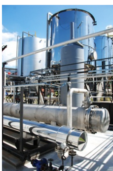
FFS De-ashing Plant
